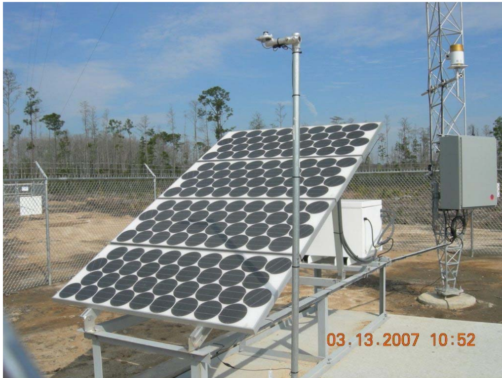
Photo 3 – Solar Power System and Instrument Enclosure
